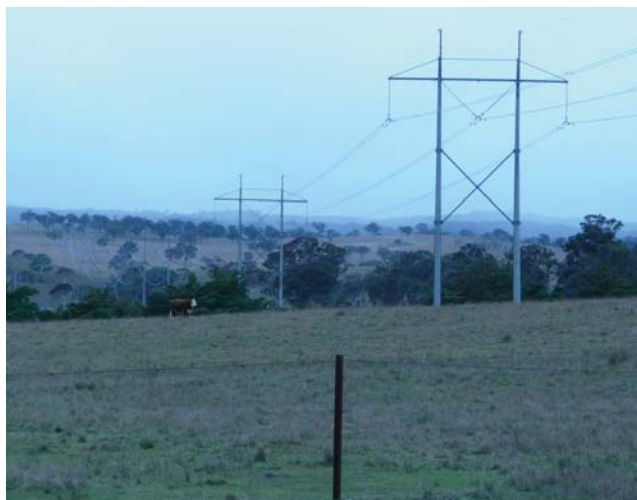
Image: A typical 330,000 volt transmission line
