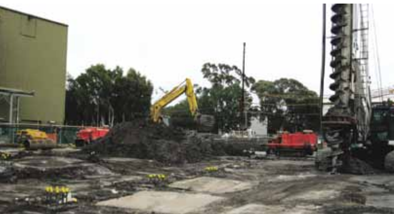
Construction is well underway on the Southern Site of the Beaconsfield West Substation Redevelopment.
