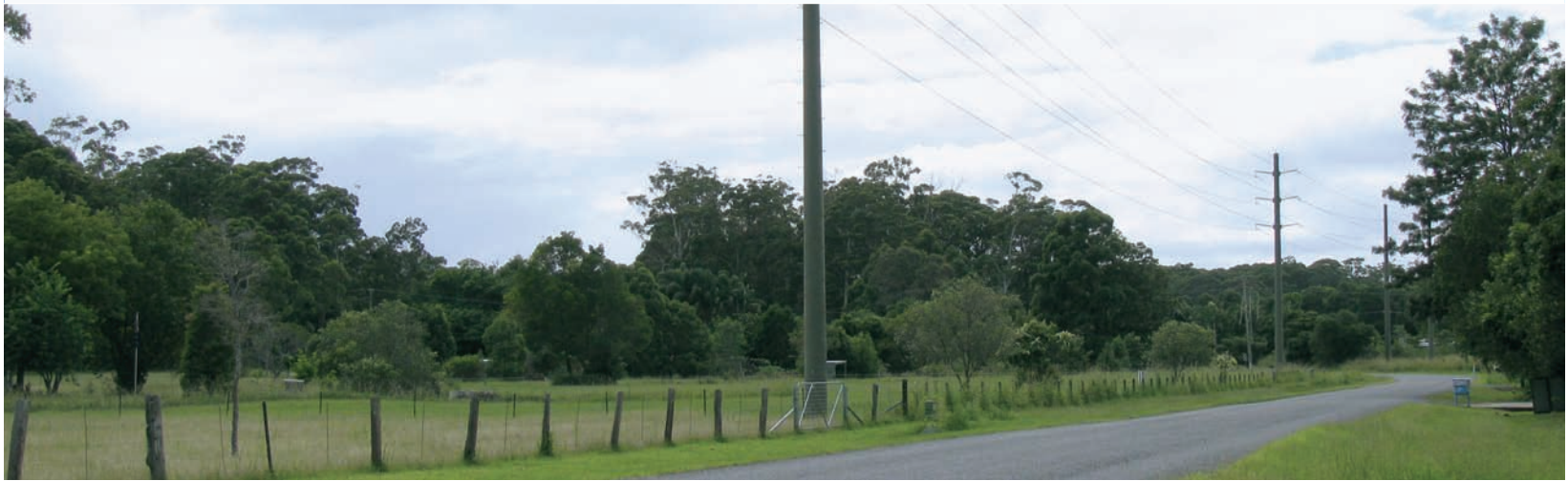
An example of a 132 kV structure, which will be used for the proposed Tomago to Stroud Project
