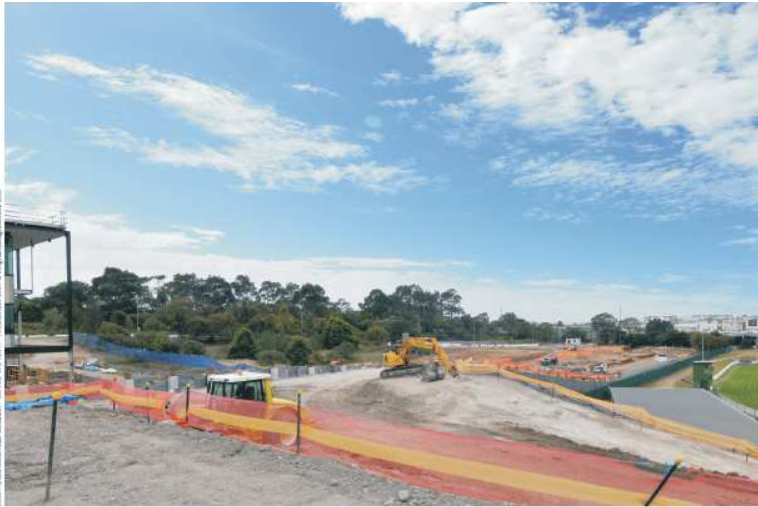
Viewpoint 2 - Existing view looking north east from William Holmes Street roundabout towards substation
