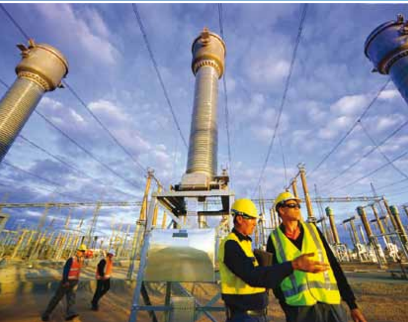
The overhead transmission line will be upgraded from TransGrid's Sydney West Substation at Eastern Creek.
