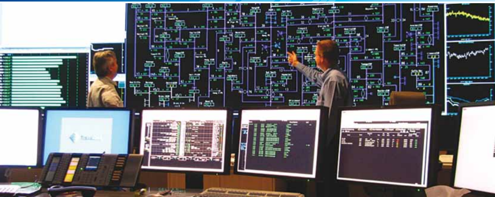
TransGrid's state of the art control room is staffed 24 hours a day, 7 days a week, monitoring TransGrid's power network and ensuring a safe and reliable electricity supply across New South Wales.
