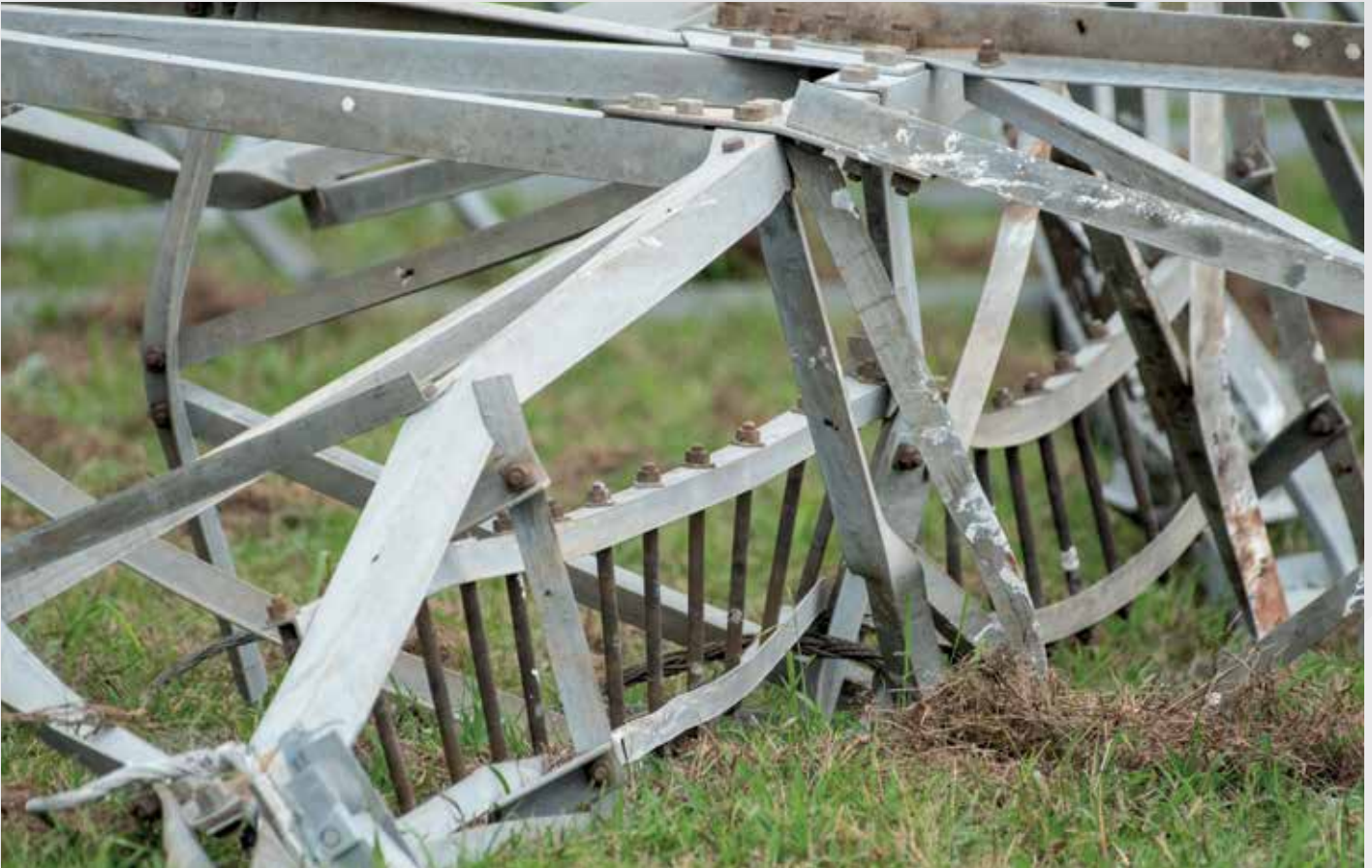
Figure 4: Transmission asset damage
