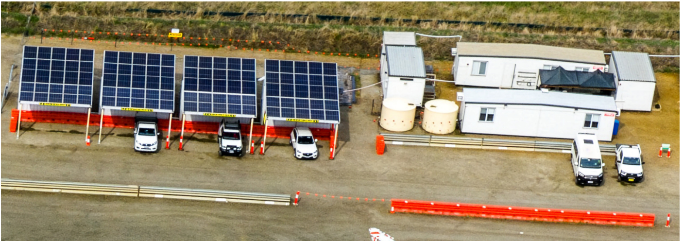
The new hybrid solar battery power supply system doubles as a handy carport for vehicles to park beneath. The solar panels are mounted on the folding roof.
