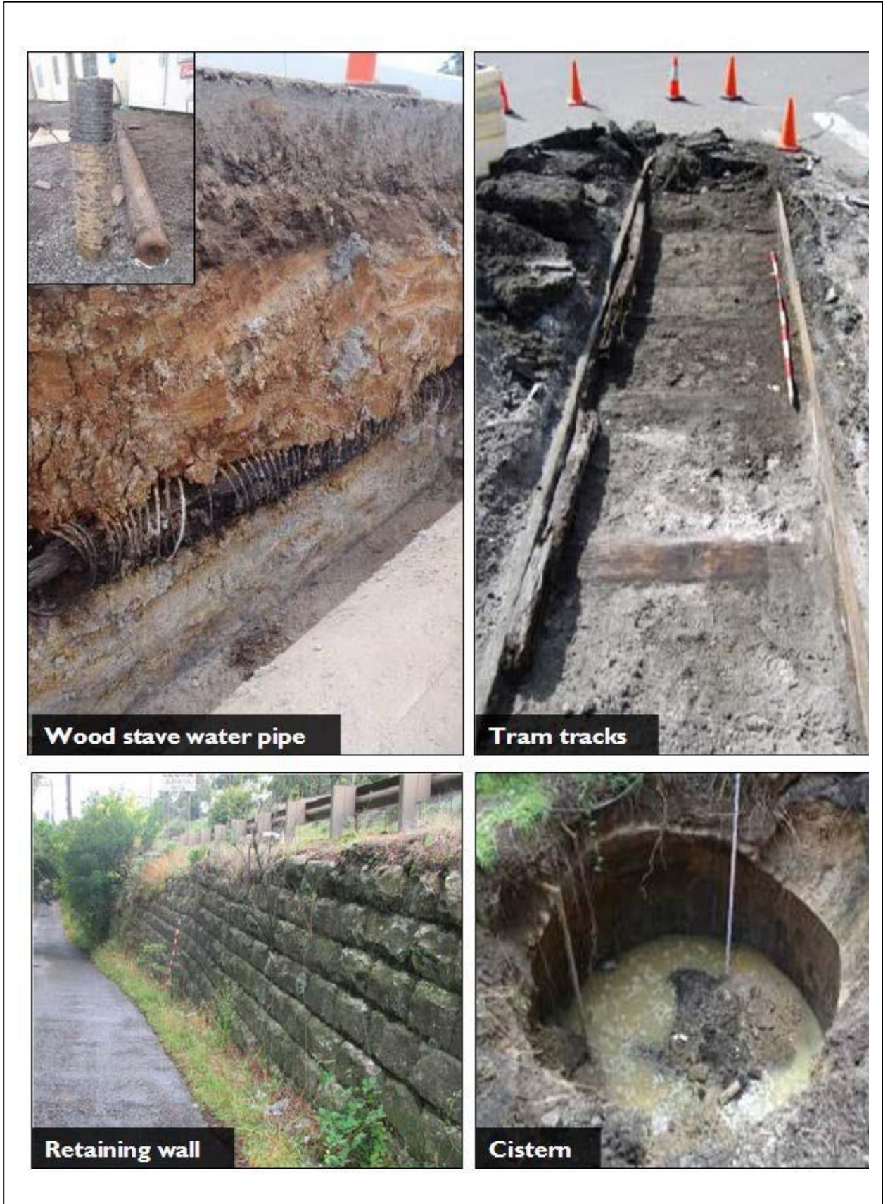
Top left hand picture continuing clockwise: Woodstave water pipe with tar and wire sealing (Horsley Drive); Tram tracks (Sydney); Brick lined cistern (Clyde); Retaining wall (Great Western Highway, Leura).
