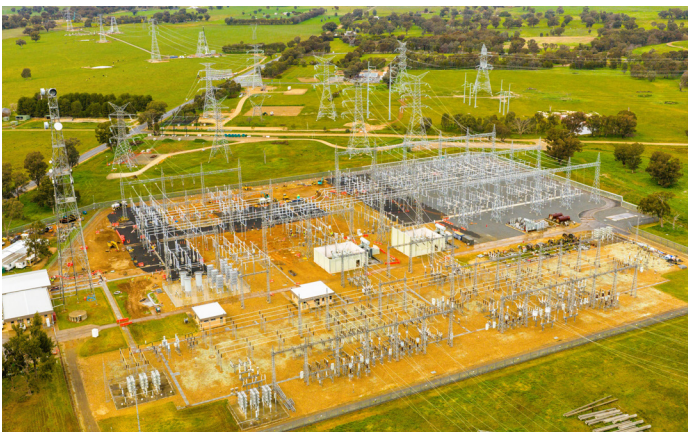
Wagga Wagga Substation where upgrade works have been completed.
