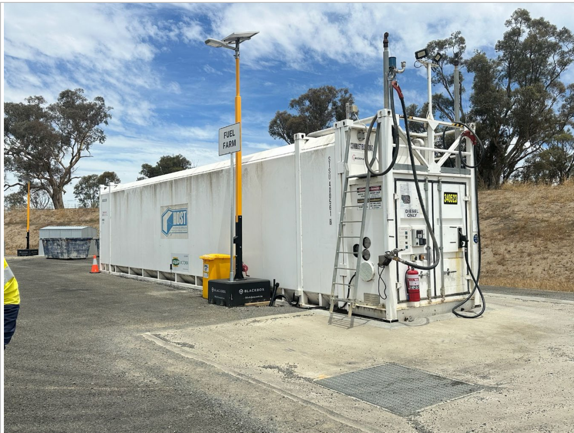
Photo 25: Double skinned tank
