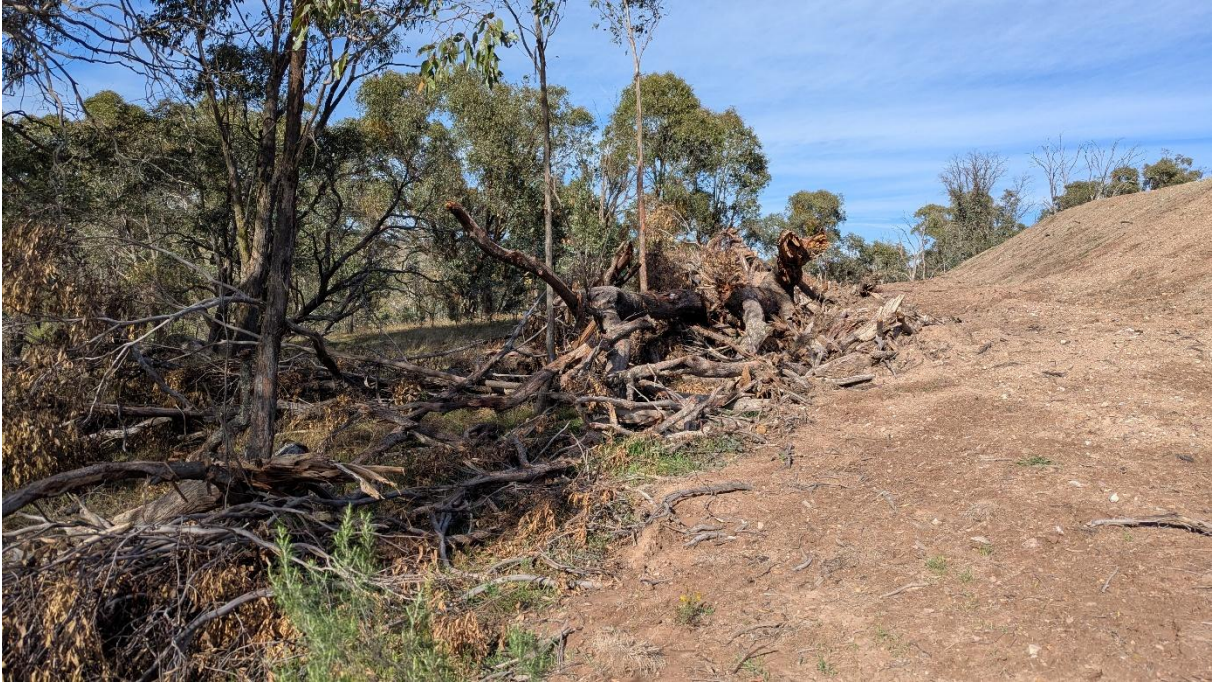
Photo 8: Coarse woody debris used to control sediment dispersal below the tower pad at Tower 55 on BY-030, showing sediment reaching the control point
