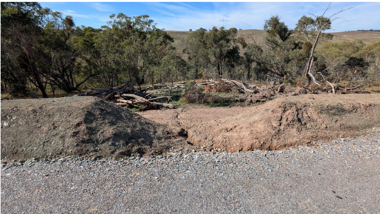
Photo 10: Drop structure constructed in the wall of tower pad at Tower 55 on BY-030 to control water flow from the tower pad
