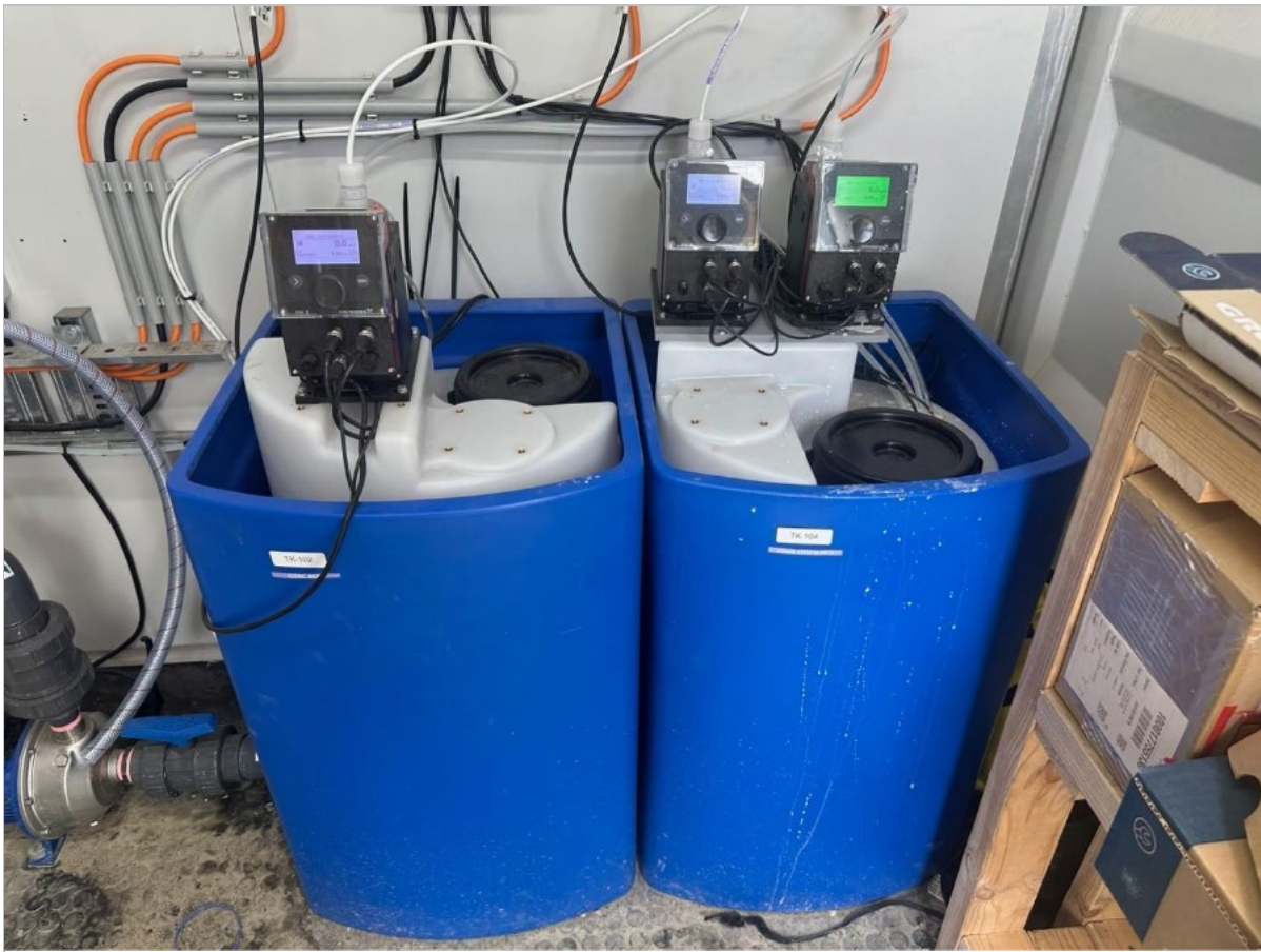
Photo 11: Camp water treatment system
