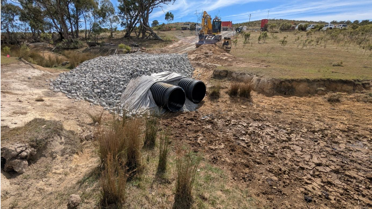
Photo 13: Downstream extent of the waterway crossing of an unnamed second-order stream in BY-040
