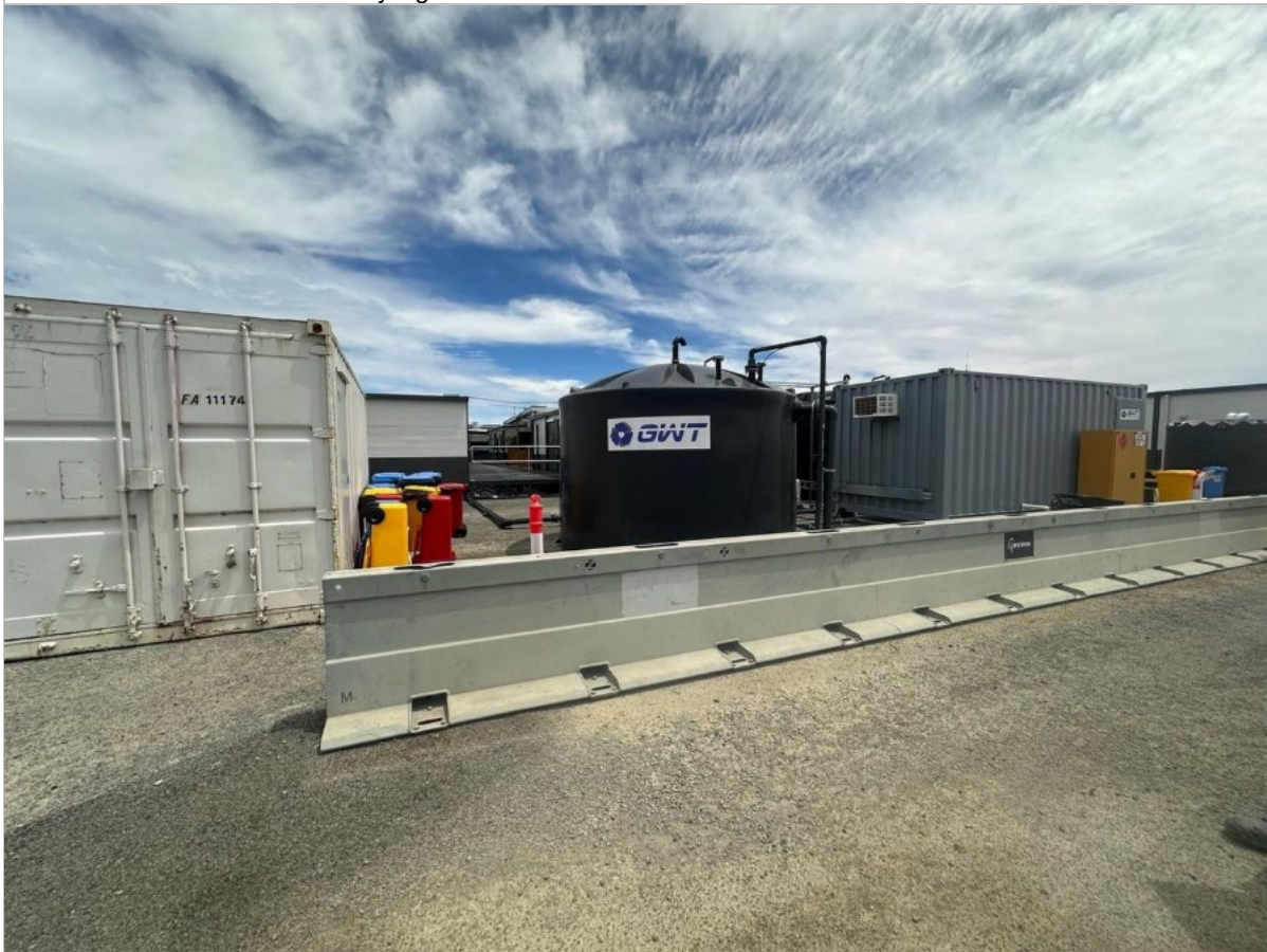
Photo 10: Water treatment system
