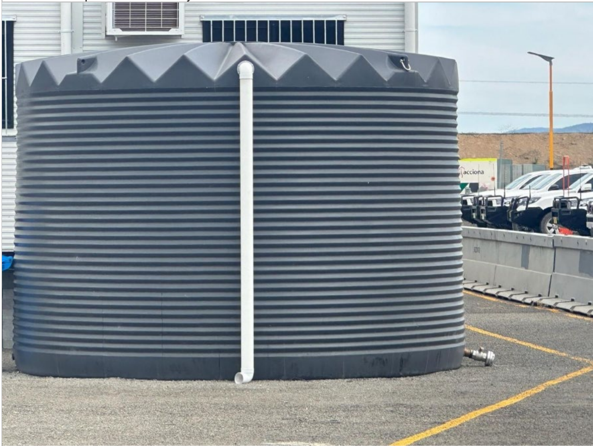
Photo 12: Fire water tank
