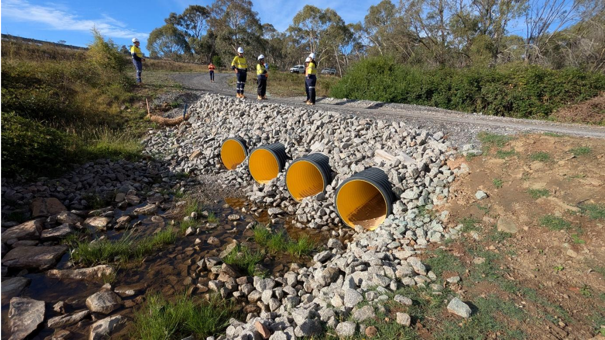
Photo 3: Downstream view of the waterway crossing of an unnamed tributary of Cowpers Creek in BY-030
