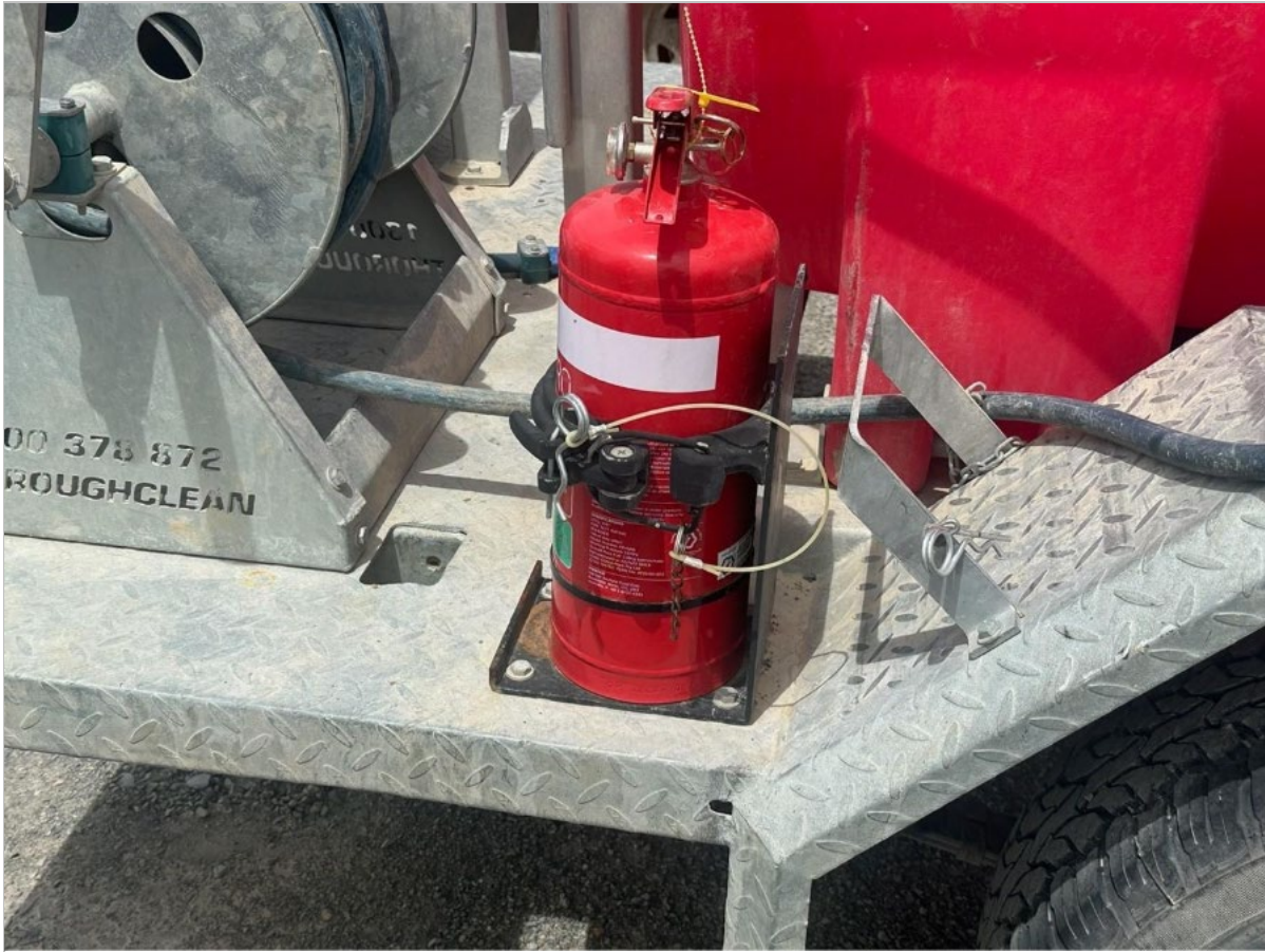
Photo 13: Mobile fire fighting equipment
