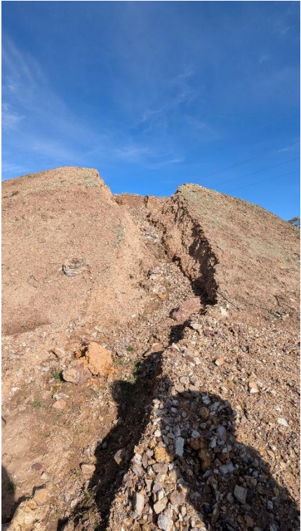
Photo 6: Wall of tower pad at Tower 55 on BY-030 showing erosion of the wall below the tower pad
