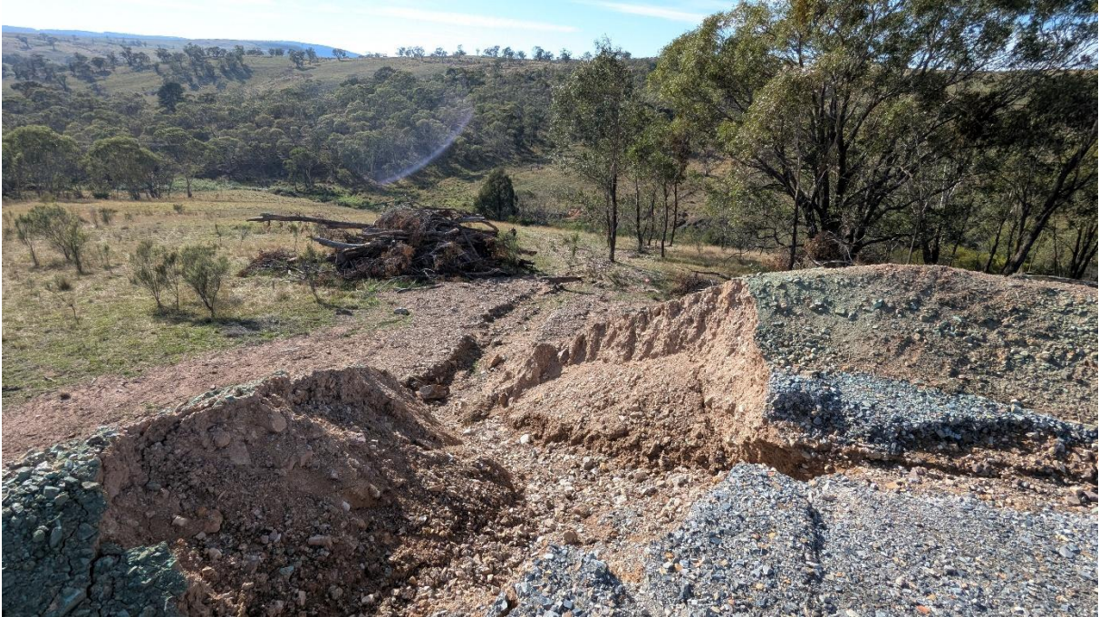
Photo 5: Wall of tower pad at Tower 55 on BY-030 showing erosion of the wall
