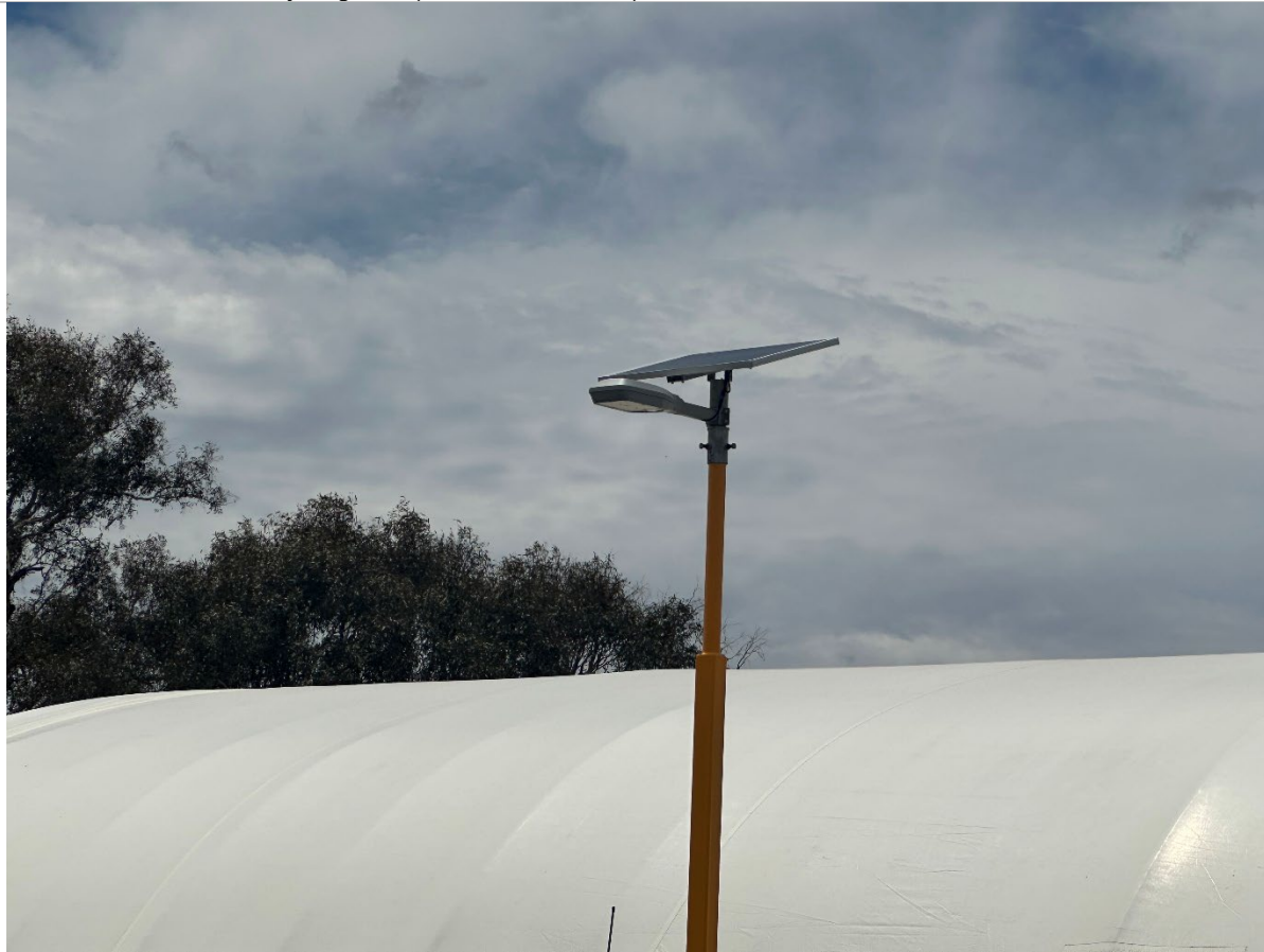
Photo 28: Low level security lighting
