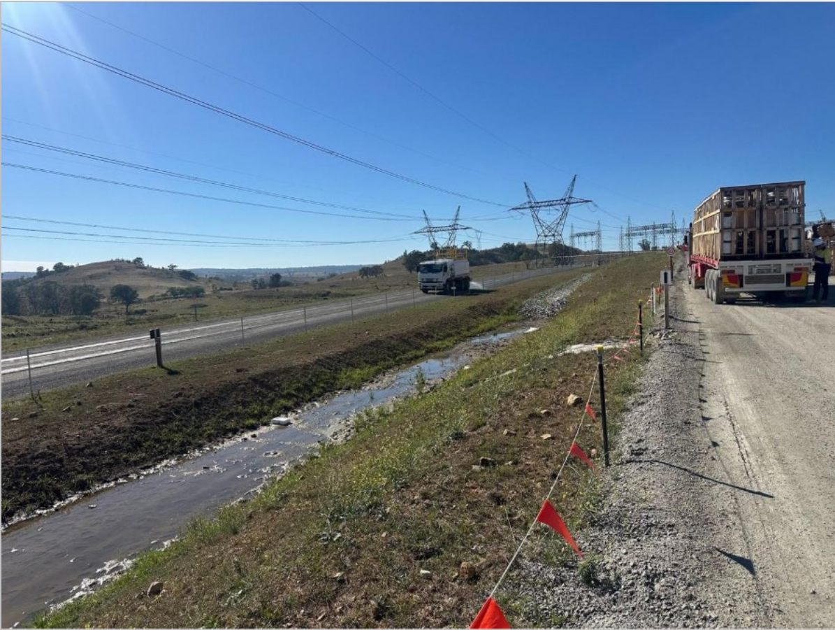
Photo 39 : Internal drainage and water cart
