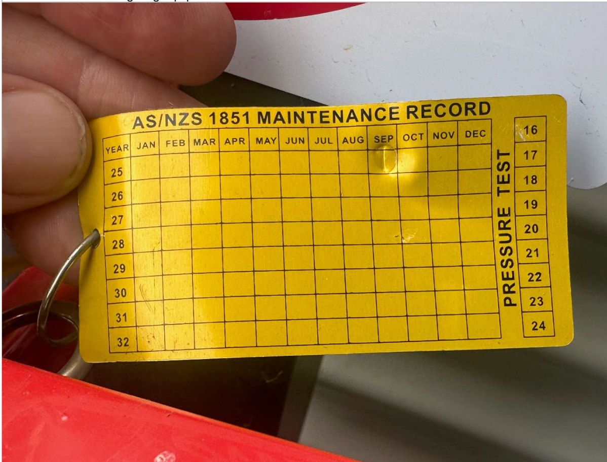
Photo 14: Fire fighting equipment test record
