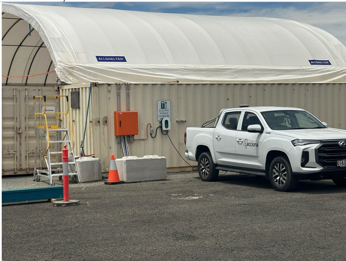
Photo 32: EV recharging station
