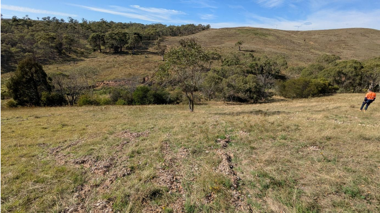
Photo 7: Sediment dispersal from erosion of the wall below the tower pad at Tower 55 on BY-030
