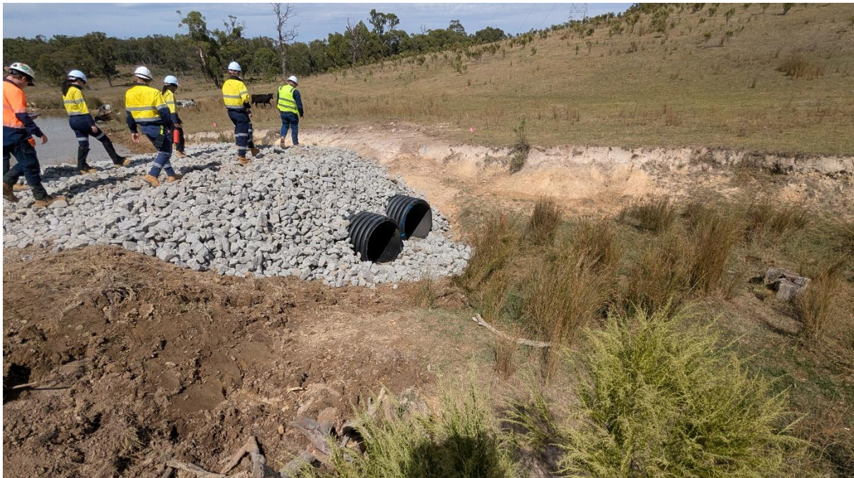
Photo 12: Upstream extent of the waterway crossing of an unnamed second-order stream in BY-040
