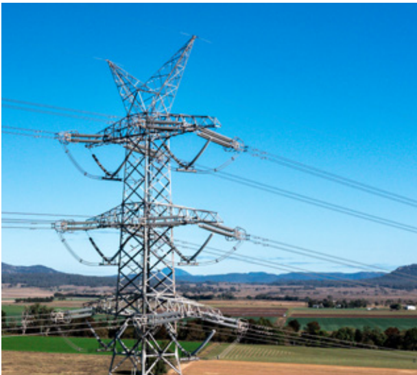
Pictured: A 500 kV transmission tower.
