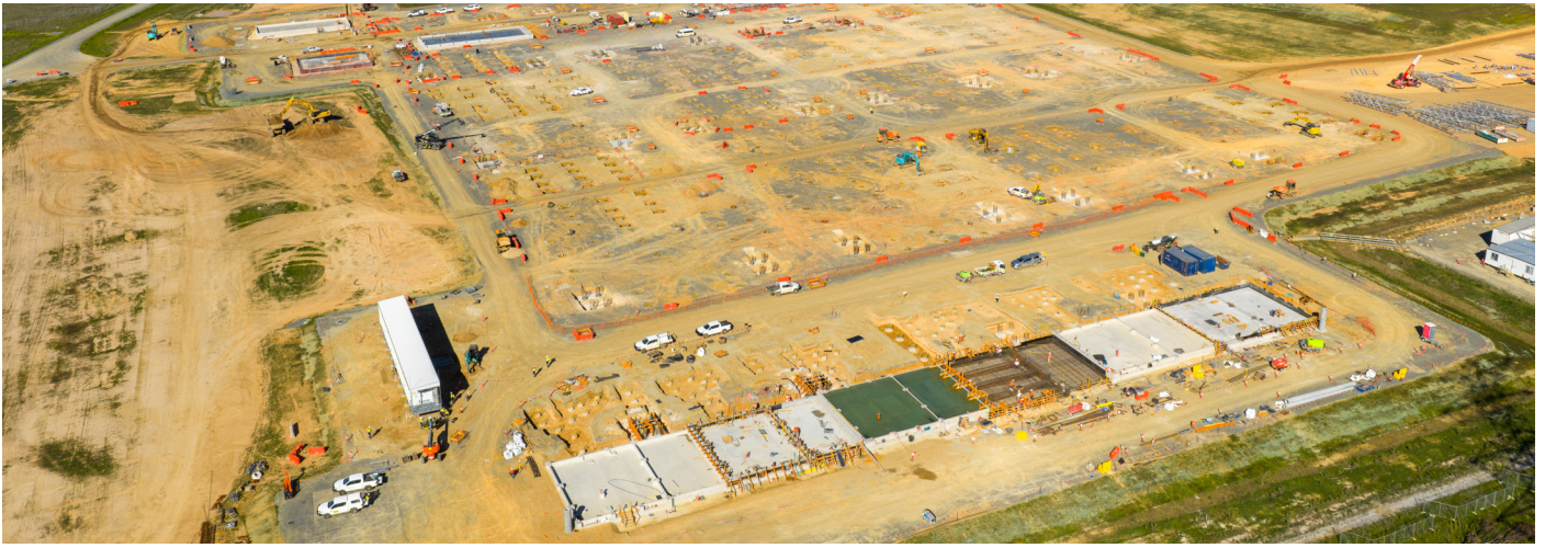
Concrete pouring of bunds is nearing completion at Gugaa Substation in readiness for transformer and reactor deliveries over coming weeks.
