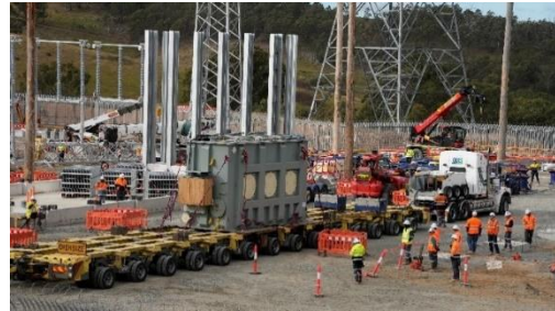
Shunt reactor arrives at Bannaby substation.
