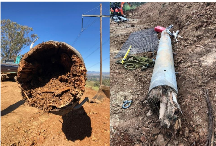
Figure 2-1: Example of wood rot on Line 86
