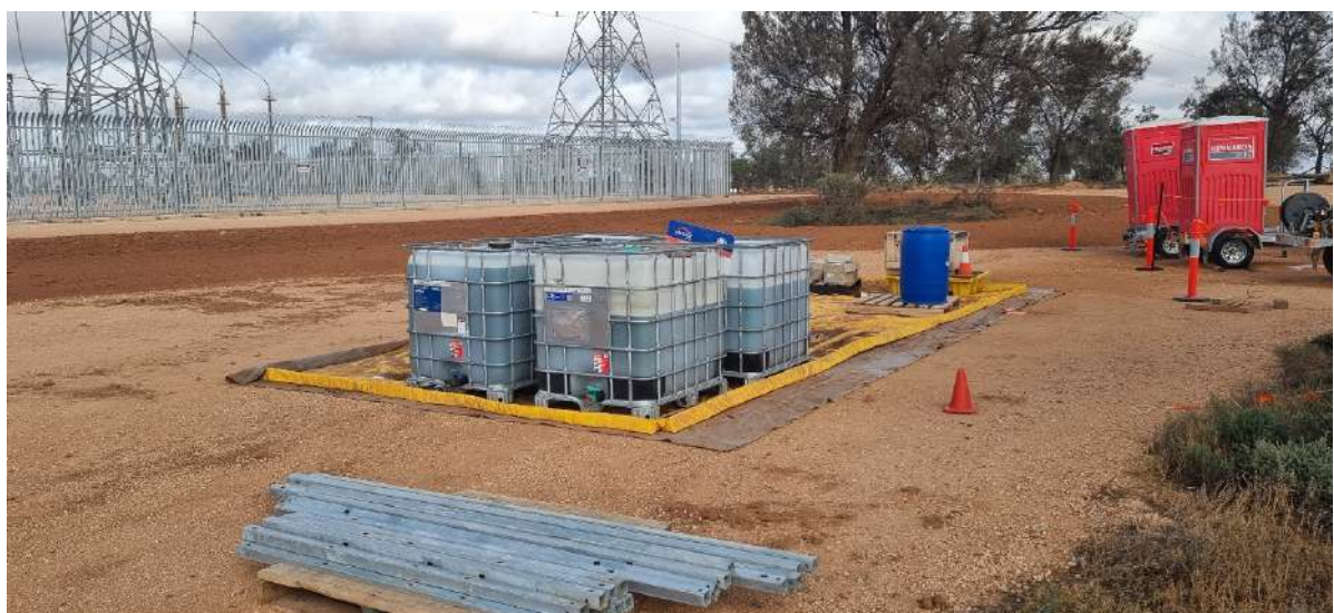
Photograph 3 – Temporary bunded hydrocarbon storage
