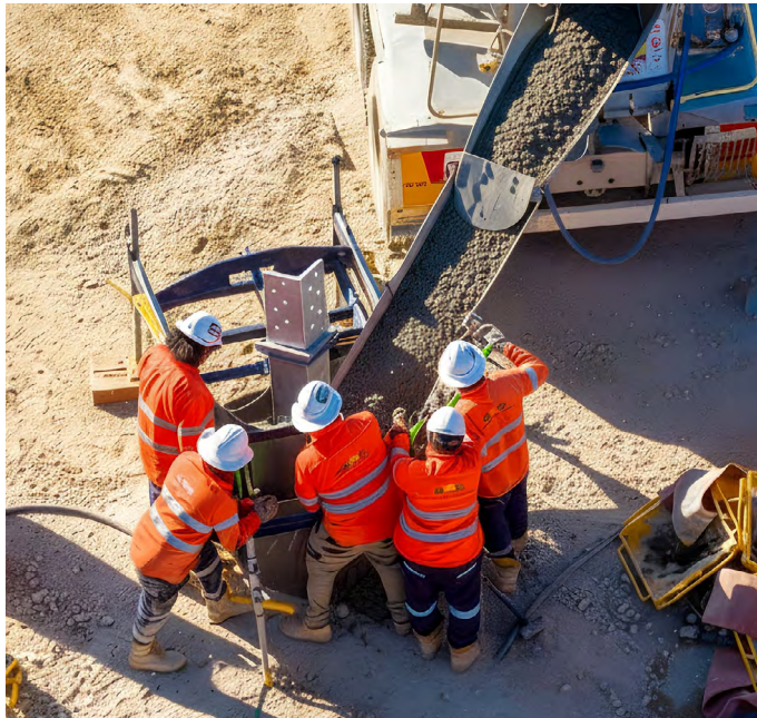
With the tower leg stub in place, the foundation pile is filled with concrete.
