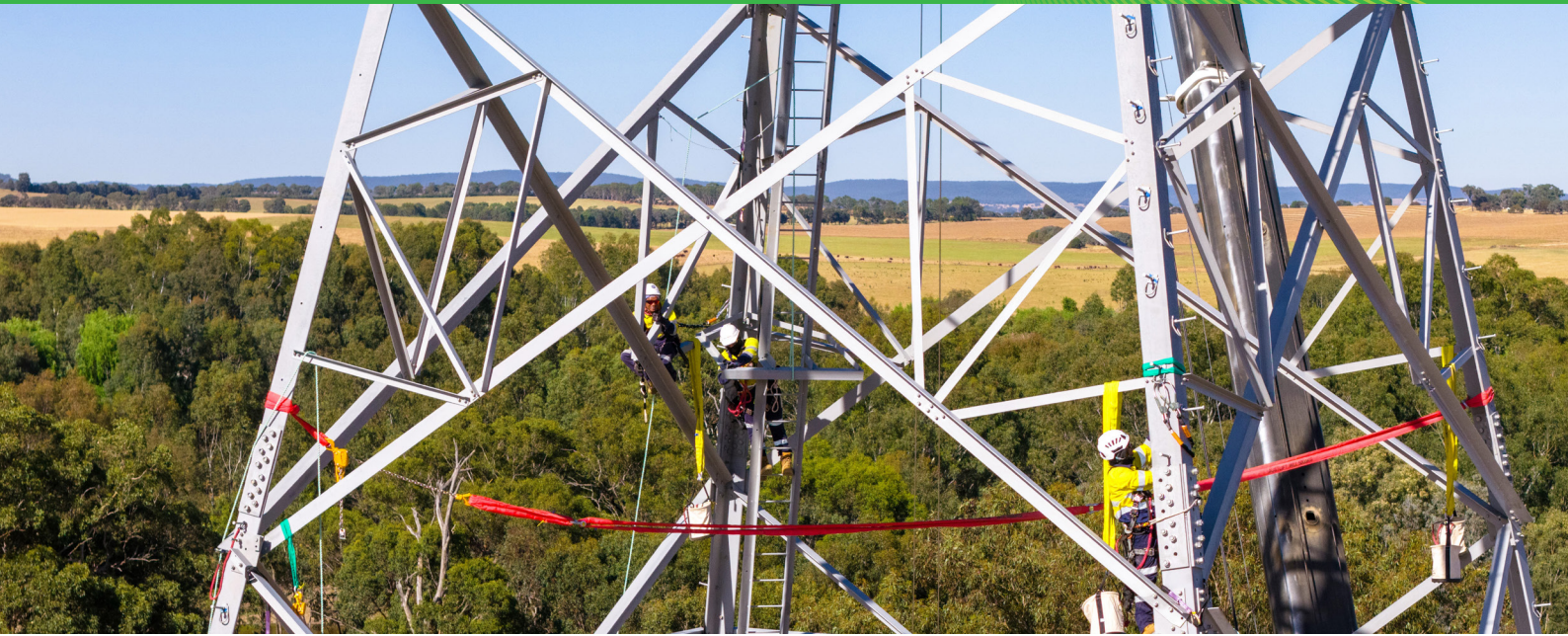
Workers in climbing safety harnesses help erect the first transmission tower on HumeLink West.
