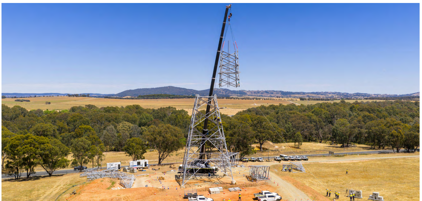
The first tower segments are lifted and bolted together during tower erection.
