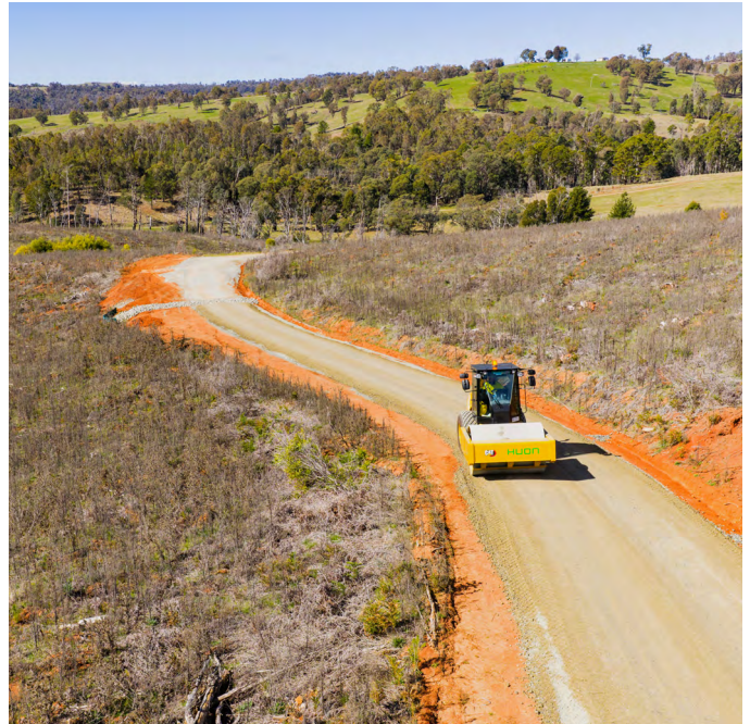
Preparing one of the tower site access tracks needed for HumeLink West.
