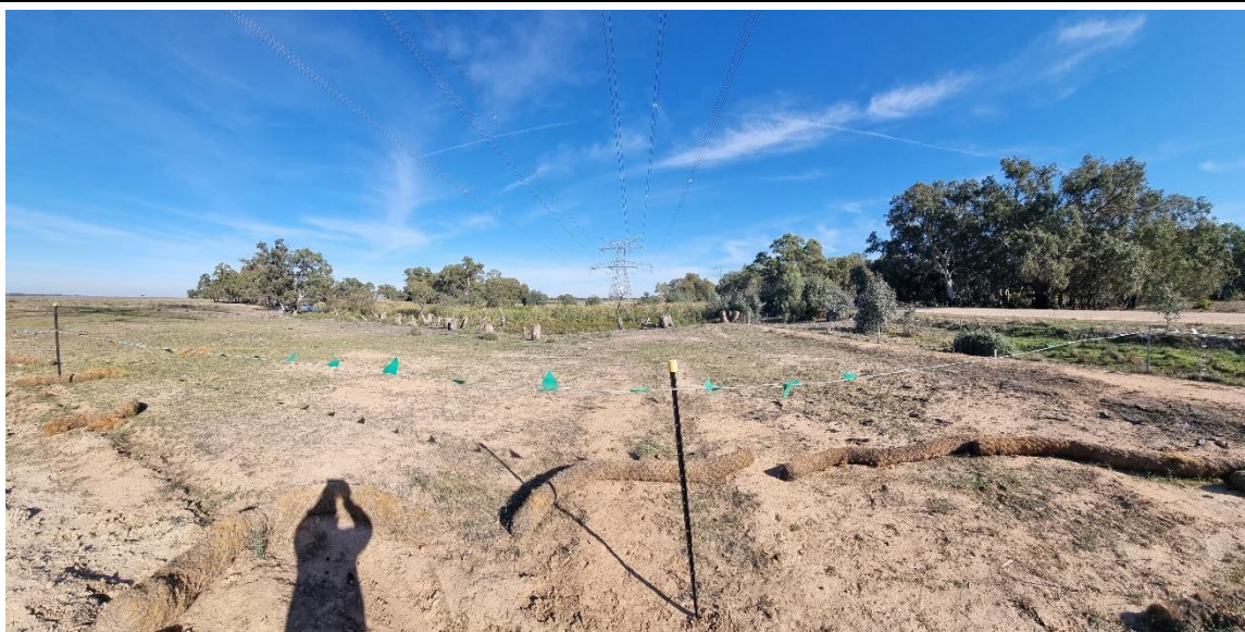
Photograph 8 – ERSED controls at Columbo Creek
