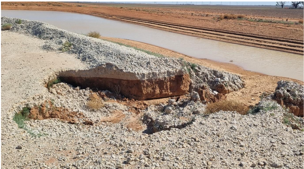
Photograph 4 – Former Limondale laydown area washout from recent storm event
