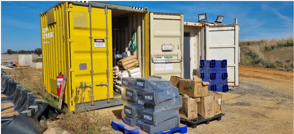
Photograph 11 – Temporary Chemical Storage Container.
