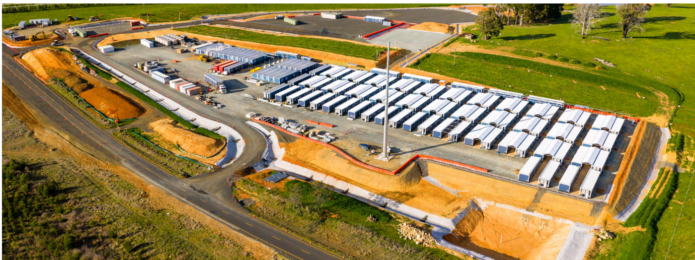
The near complete Kunama worker accommodation facility showing associated road widening and upgrade works along Green Hills Access Road.
