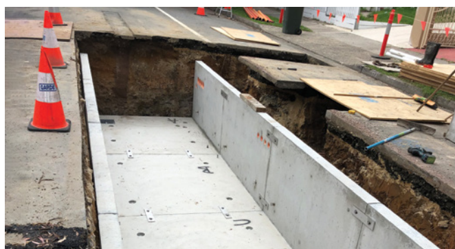
Joint bays are installed about every 900 metres along the cable route, and are constructed wider than the trench
