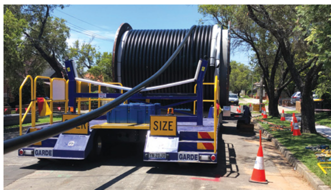
A large truck will be parked in the streets when cables are pulled from a cable drum and fed into the conduits in the trench
