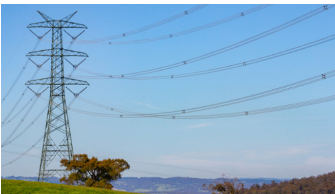
Image 1: Example of a 500 kV transmission line structure.
