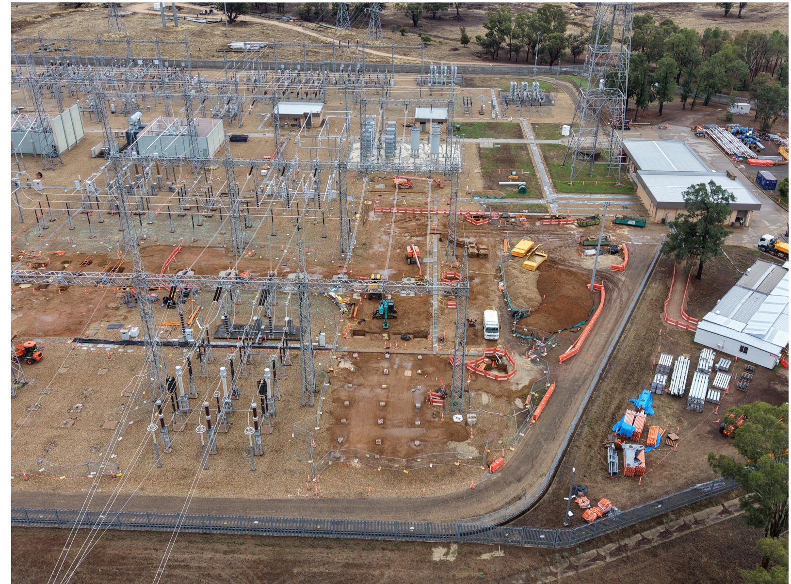
Image of current construction activity at Wagga 330kV substation as part of EnergyConnect and HumeLink work
