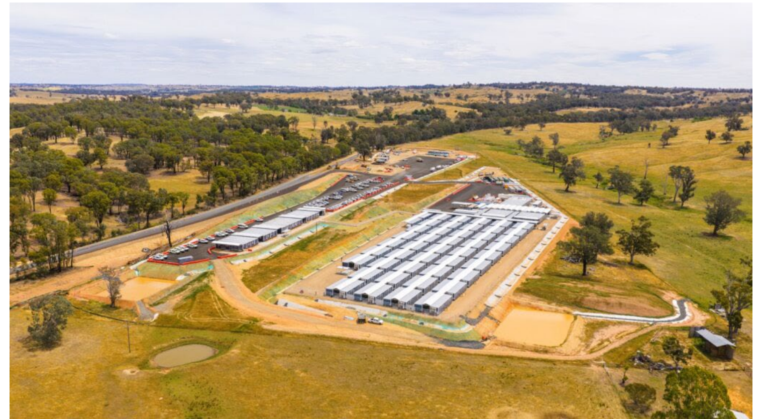
Image of worker accommodation camp and construction laydown area at Tarcutta for the HumeLink project
