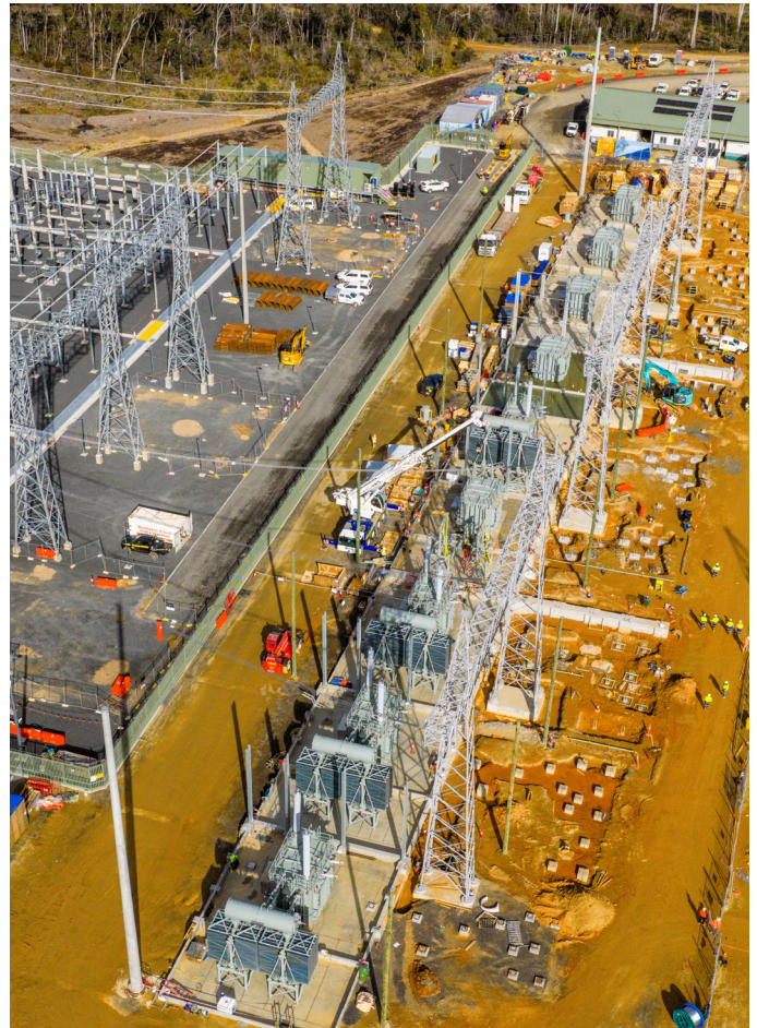
The nine recently installed power transformers at Maragle Substation.
