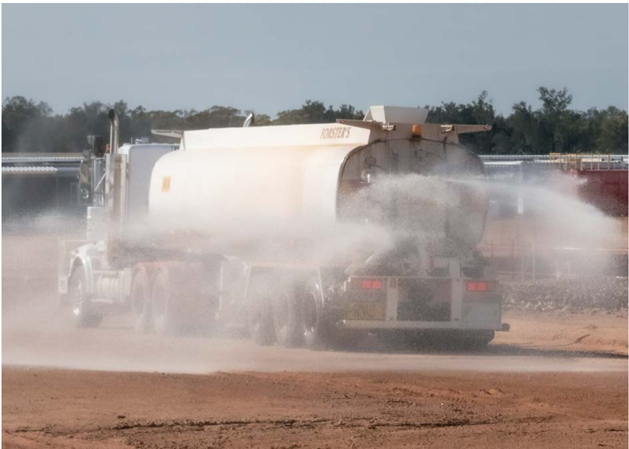
Pictured: A water cart is used to control dust on construction sites.
