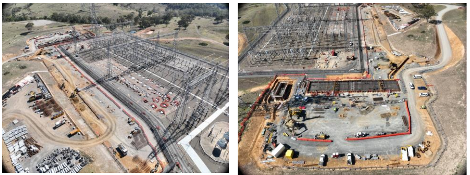
Images: Bannaby substation
