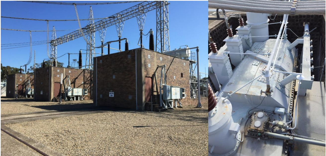
Figure 2-3 – Examples of the condition of Sydney East transformers
