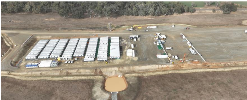
The accommodation modules are now in place at the Adjungbilly worker accommodation facility (May 2025).
