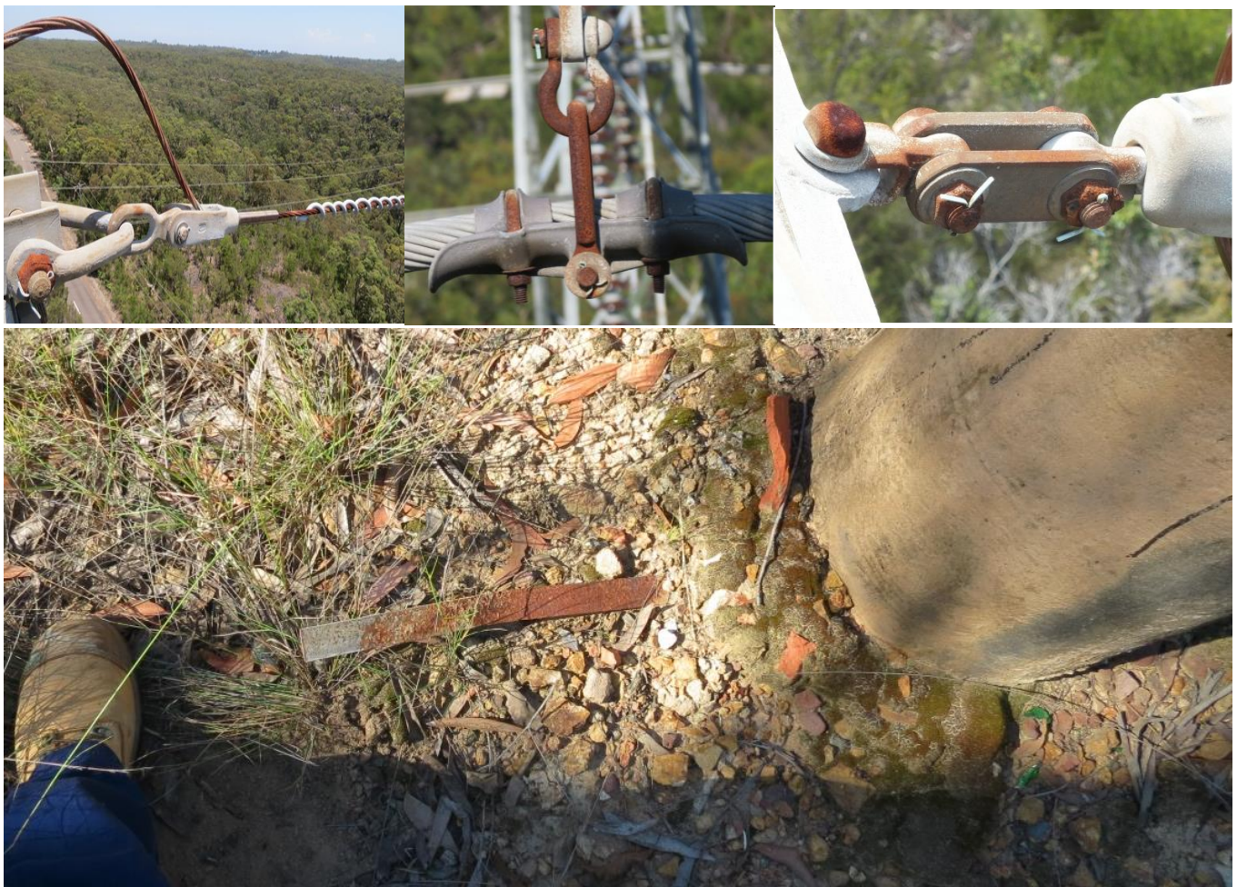
Figure 2-2 – Corroded components of Line 959/92Z
