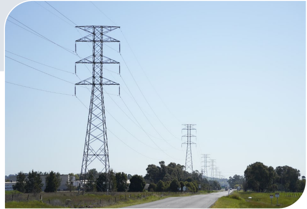
Figure 2: Example of a free-standing 330 kV transmission line structure.
