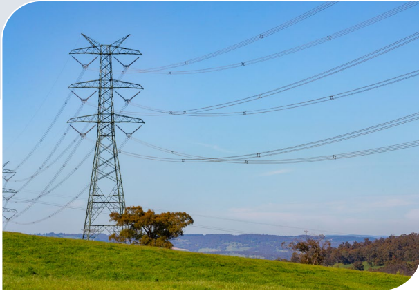
Figure 1: Example of a free-standing 500 kV transmission line structure.
