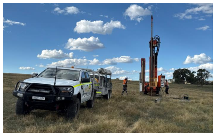
A geotechnical inspection using a borehole drill to collect soil samples near Biala.
