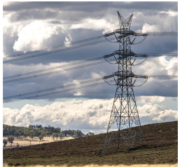
Pictured: EMF are produced wherever electricity is flowing.
