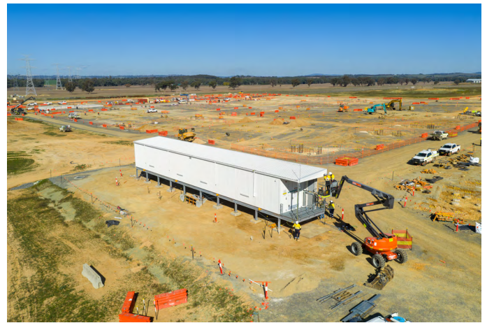
The auxiliary services building has been installed at Gugaa Substation.
