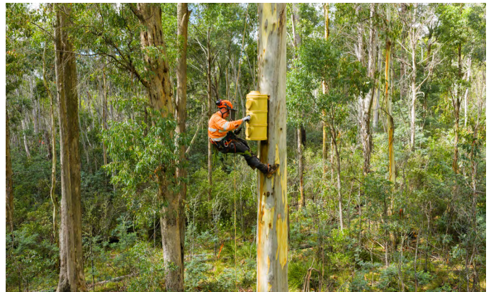
A worker installs a bird nesting box adjacent to the HumeLink West corridor.
