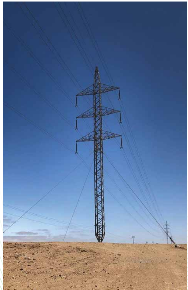
Guyed transmission tower
