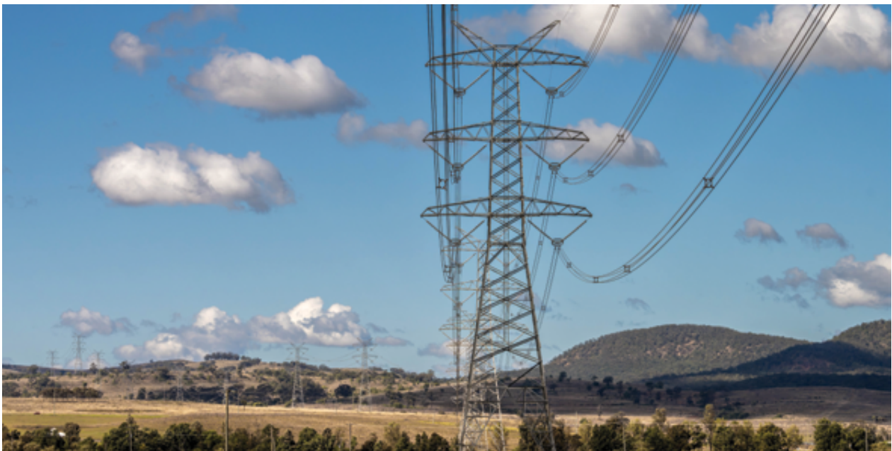
Pictured: Example of a 500 kV transmission tower.
