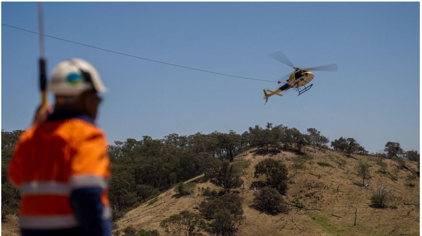
An example of a similar helicopter stringing set up as will be used on HumeLink East
