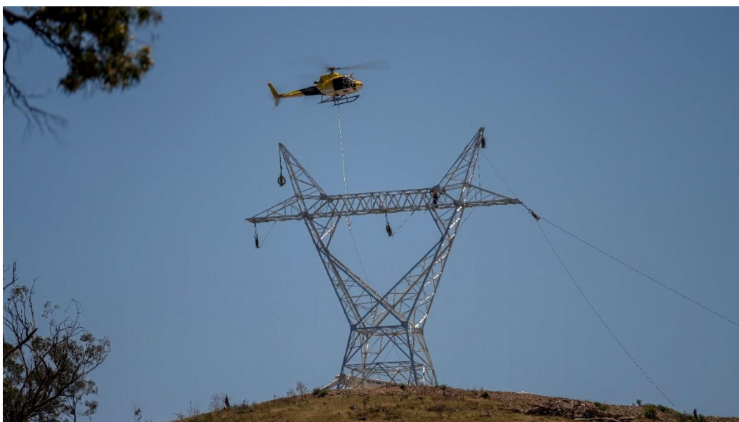
An example of a similar helicopter stringing set up as will be used on HumeLink East
