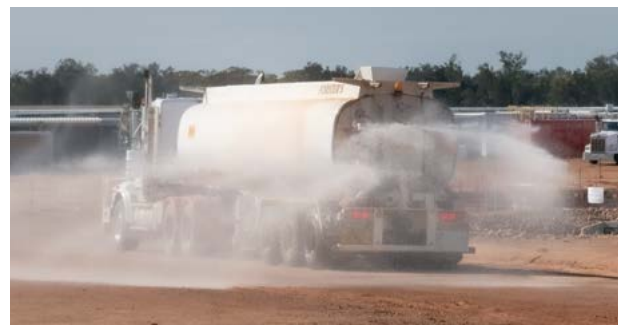
Pictured: A water cart is used to control dust on construction sites.
