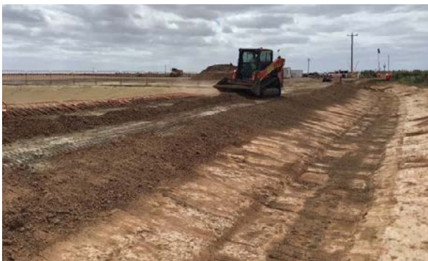
Pictured: Swale drain, similar to what may be constructed on HumeLink, used to manage surface water flows.
