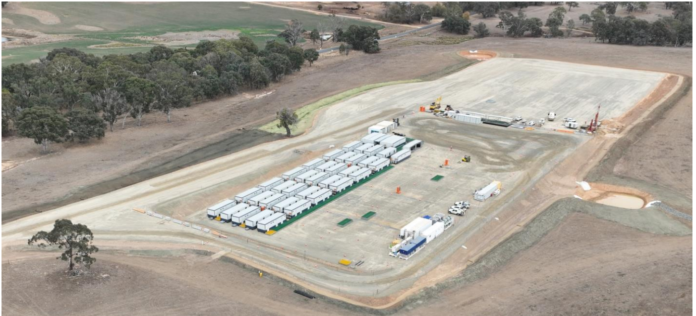
An aerial view of the Adjungbilly worker accommodation facility taking shape (May 2025).
